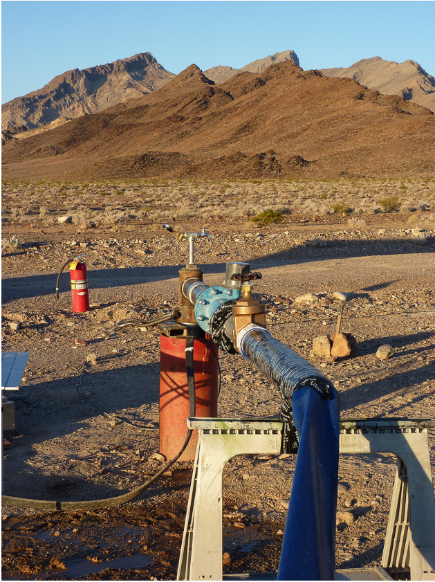
Figure 5. Possible drilling site near Death Valley, California, on the eastern flank of the Funeral Mountains. A consortium of interests, including the U.S. Department of Energy, U.S. Geological Survey, Inyo County, California, and the Hydrodynamics Group, LLC, drilled a well (BLM-1) to 883 m depth through a range of sedimentary and volcanic lithologies and conducted two hydrologic pump tests. The underlying carbonate aquifer contains anoxic thermal water (58 °C) and abundant sulfate-reducing bacteria including Candidatus Desulfurudis sp. and Desulfotomaculum spp. (Thomas, 2013).
