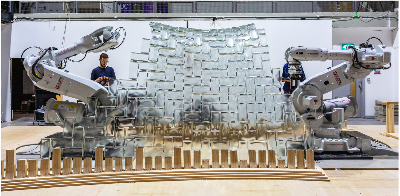
16 LightVault constructed live during "Anatomy of Structure: The Future of Art + Architecture" exhibition at Ambika P3 gallery in London, UK
