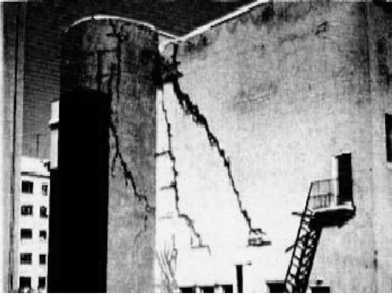
Figure 5: Structural Damage in Siberia
