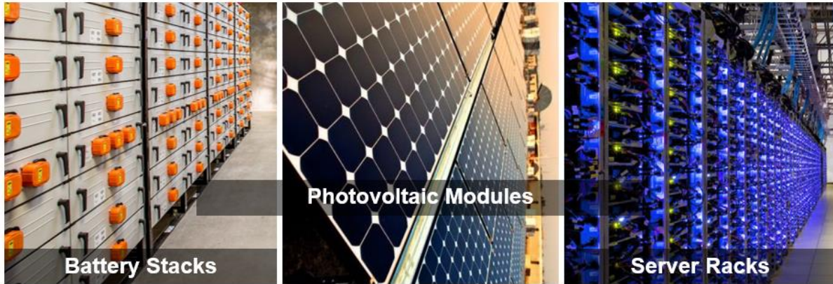
Fig. 3: Battery stacks, photovoltaic modules, and server racks all comprise a large number of modular units functioning together at the grid edge.
